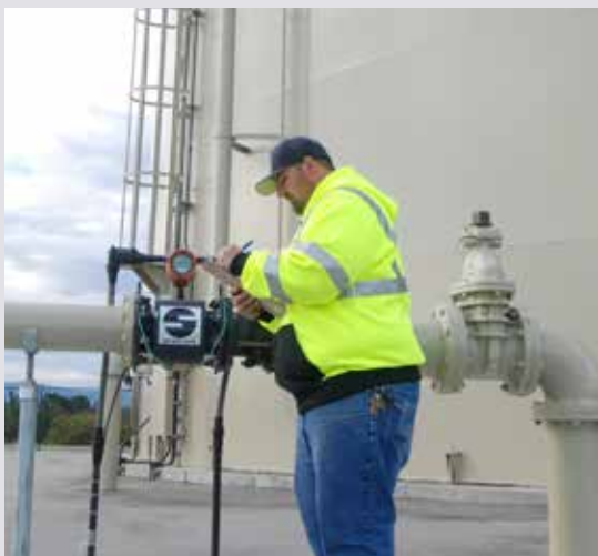
Operator inspecting and monitoring the flow meter at one of the District's reservoirs
